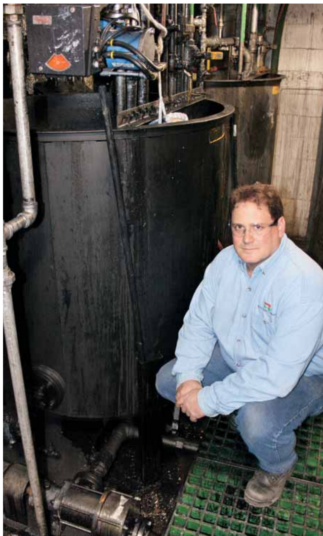
Tim Kreitz, project engineer at Rock-Tenn's St. Paul Paper Mill, kneels next to a new eccentric disc pump.
